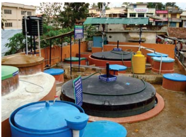
Waste to electricity plant
